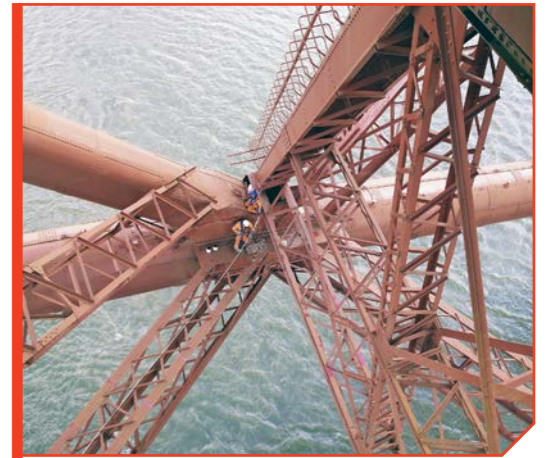
Looking down from the under-track catwalk, a pair of abseilers are dwarfed by the massive 12ft diameter riveted steel tubes. NIGEL HARRIS.
