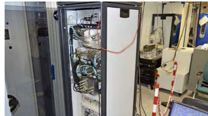
Left and above: HCI's system integration laboratory at James Forbes House in Southwark enables the offline testing of ETCS and ATO equipment using real equipment and a Class 700 simulator. PAUL STEPHEN.
