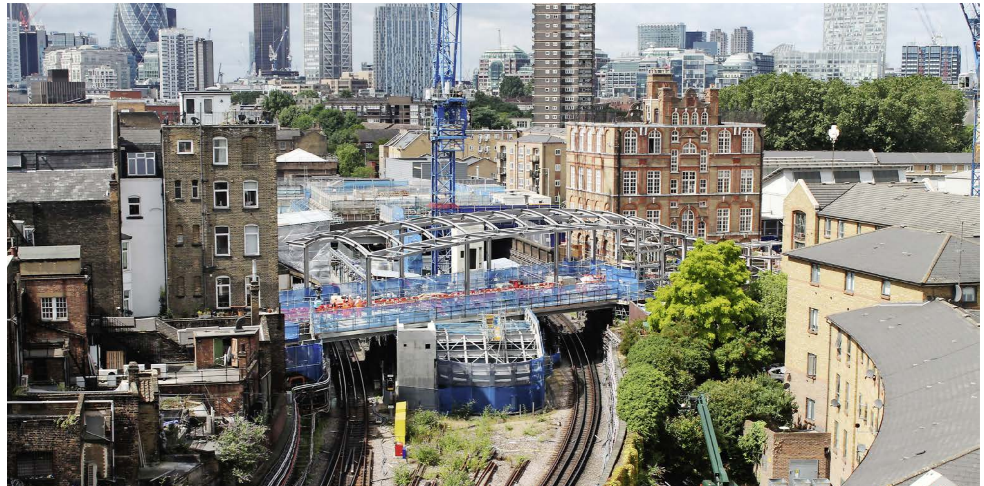
The steel frame for Whitechapel station ticket hall is being installed above operational platforms for London Overground and Underground. The significant level of risk management and stakeholder engagement required here represents one of the Crossrail project delivery partners' greatest challenges, but also successes, says Bechtel's Bill Tucker. CROSSRAIL.
