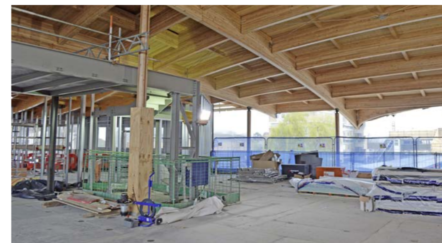
The view at concourse level on March 24, prior to interior fit-out. The main timber roof beams are 45 metres long, which is the equivalent of four London buses end to end. The new concourse measures 1,500m 2 (the size of six tennis courts). PAUL STEPHEN.
