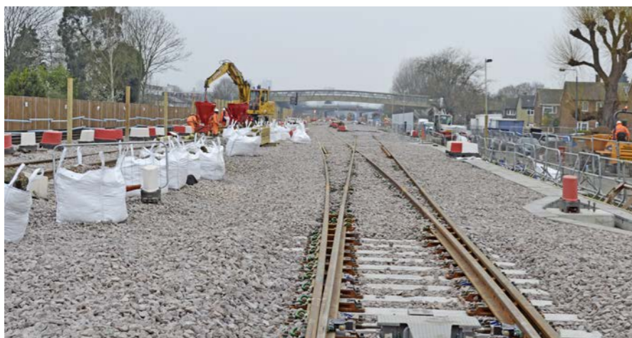
A high-speed crossover has been built at the western end of the station, with the concrete plinths for overhead line equipment visible on the right-hand side. Contractors are also erecting separation barriers between the two Crossrail tracks and those of the North Kent Line. This is required because Crossrail utilises overhead electrification and Automatic Train Control (ATO) that both require different competencies for track workers than those working with the third rail and conventionally signalled adjacent North Kent Line tracks. PAUL STEPHEN.
