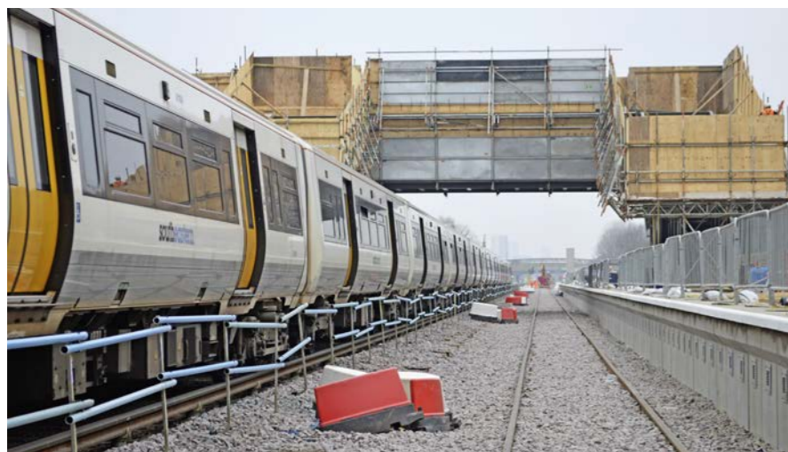
A Down Southeastern service occupies Platform 2 at Abbey Wood on March 24, demonstrating the close proximity of the fully energised North Kent running lines to the island platform constructed for Crossrail to the right. The Crossrail tracks were due to be tamped by the end of April, ahead of the installation of signalling and communications equipment. PAUL STEPHEN.
