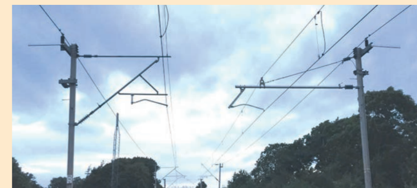
CLEver Cantilever installed in the product acceptance trial. ALSTOM.
